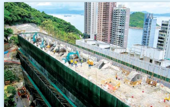
位於加惠民道的堅尼地城舊警察宿舍A座現正進行拆卸工程。 Demolition works of Block A of Kennedy Town Police Quarters at Ka Wai Man Road are in progress.
